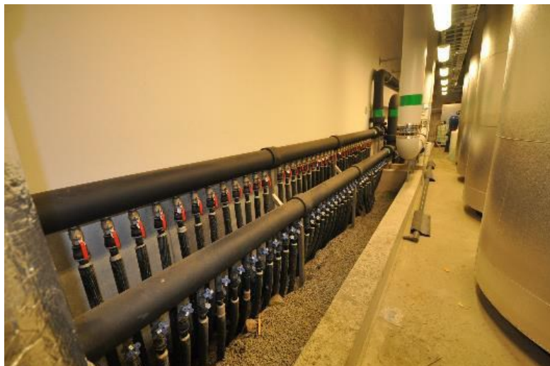
Figure 70: Piping to Boreholes in Energy Central at demo [14]
